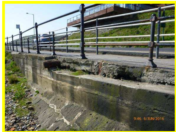
Missing coping blocks (/C0704C06)
