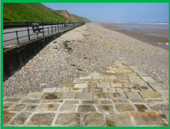
View looking northwest. High beach levels. Open joints to lower section of masonry access ramp (/C0702C04)
