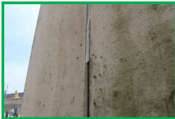
Loose and missing flexible joint sealant (/C0506C01)
