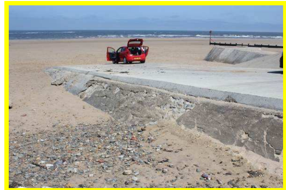
South eastern access ramp. Loss of concrete render exposing grouted stone fill beneath concrete deck slab (/C0602C01)
