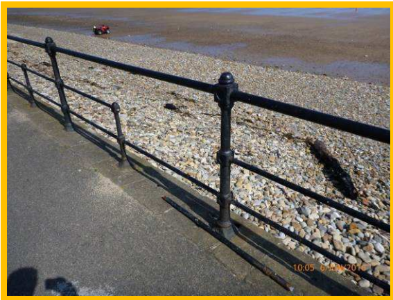
Local damage to pedestrian guardrail (/C0702C04)
