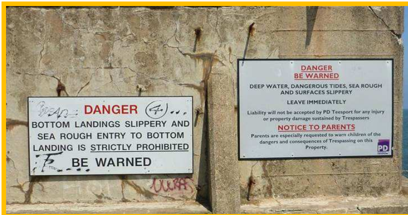
Warning signage (/C0506C01)
