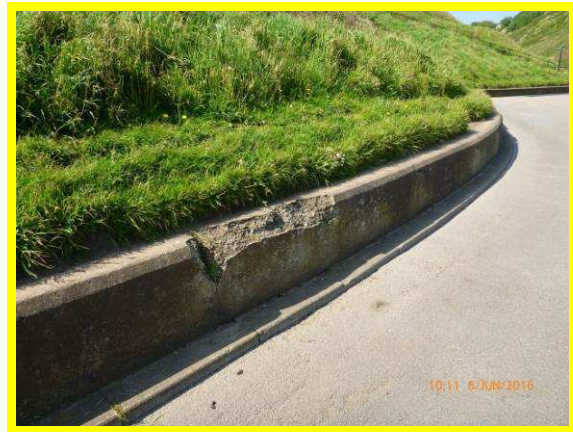
Local damage to concrete wall (/C0702C04)
