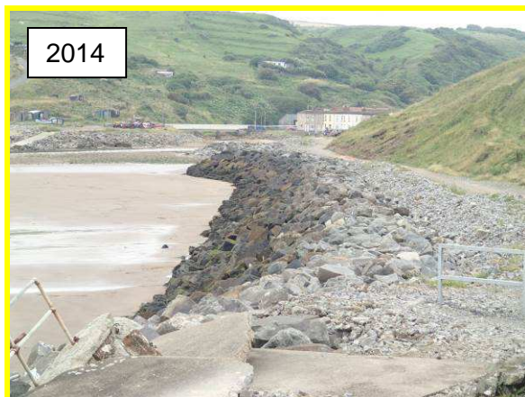
General view of revetment looking from Jetty towards village in 2014 (Asset Ref No. 1221D901D0202C01)
