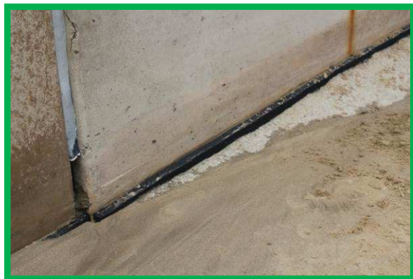
Missing flexible joint sealant in vertical joint. No sealant in horizontal joint – black filler board visible (/C0602C03)
