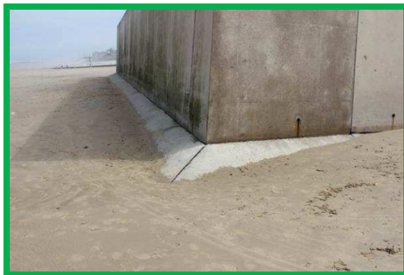
Exposed concrete apron – no sealant in joints – black filler board visible (/C0602C03)
