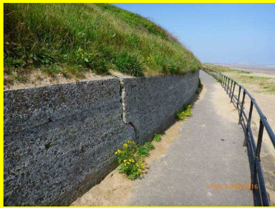
Crack in wall – no apparent change (/C0702C03)
