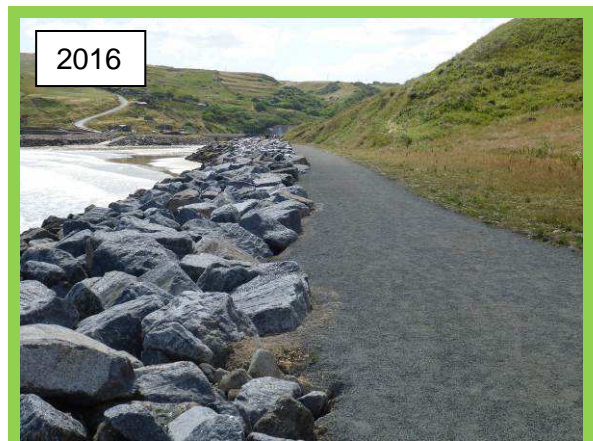
General view of modified revetment and surfaced path looking from Jetty towards village in 2016 (Asset Ref No. 1221D901D0202C01)
