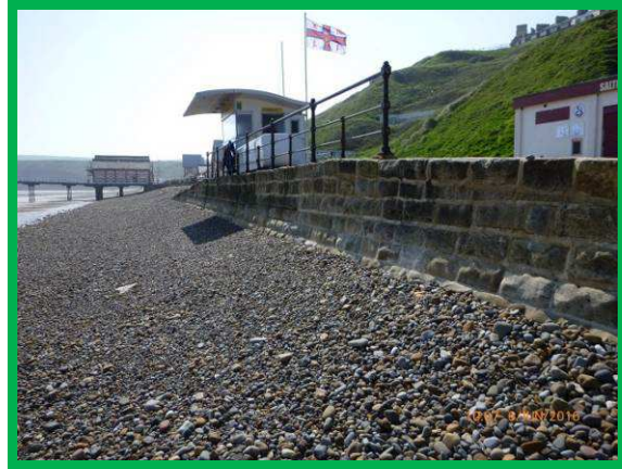
Exposed masonry at slipway (/C0702C04)
