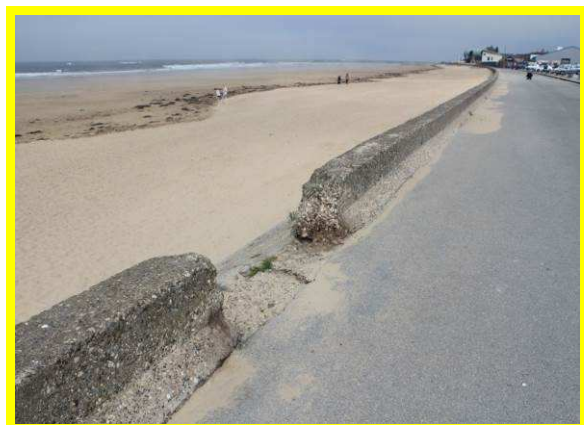
Gap in concrete wall (/C0601C01)
