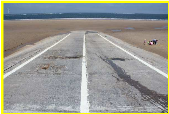
Cracking and local damage to surface of RNLI slipway (/C0602C02)
