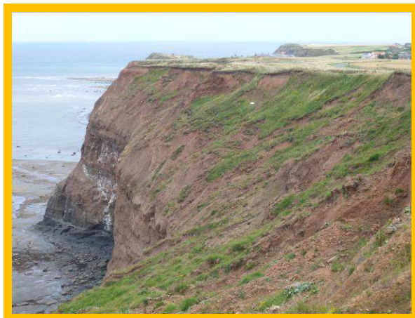
E58/1 to E/59/6 Soft, slumping, upper till resting upon harder rock (Partly Active)
