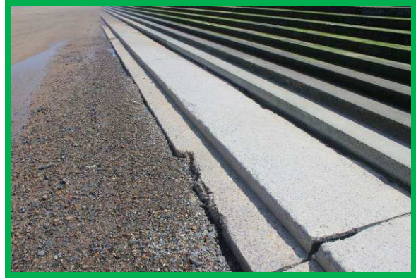
Local minor damage to lower in situ concrete toe section where exposed (/C0602C01)
