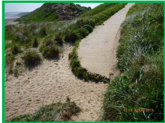
Exposure of timber piles at foot of concrete footpath (CBU E52/6)
