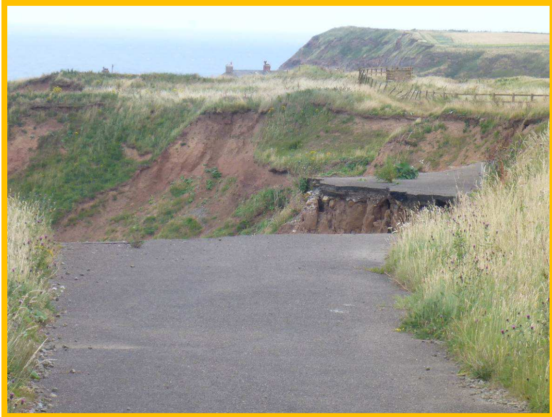
E59/3 and E59/4 Loss of road due to ongoing erosion at Cowbar Lane
